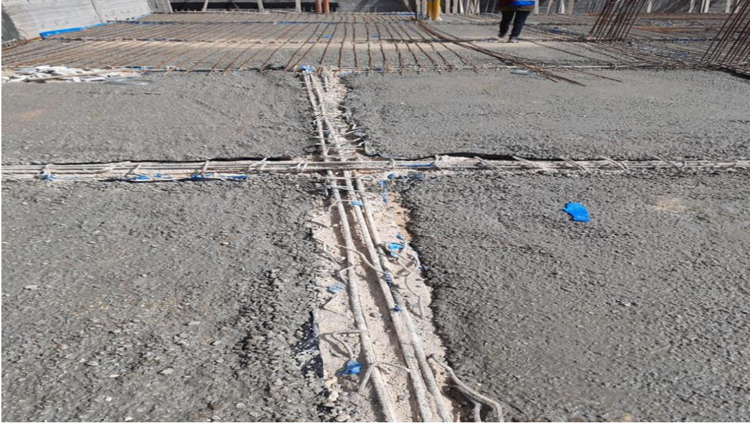
Defected Works- QC Report 2104
