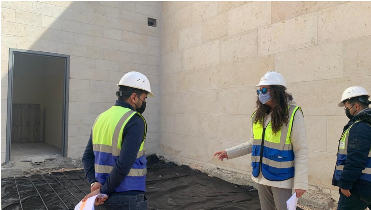
The team inspected the ongoing work at the walkways around the building
