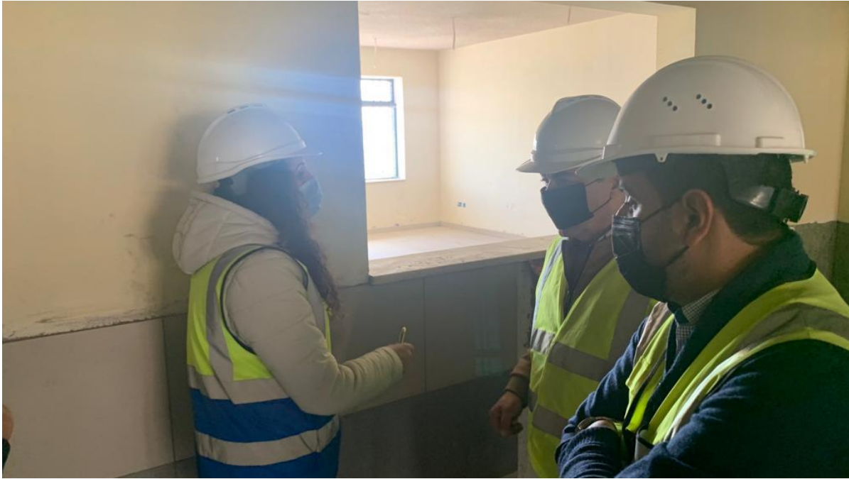
The team inspected the tile cladding at corridors and the relation with the sills of internal windows and the height of lockers there
