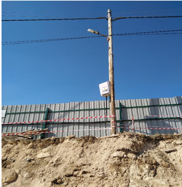
Figure #2: A power pole was observed at the top edge of excavation in unsafe condition. Photo credit: Odai Tawalbeh, 11/18/2020
