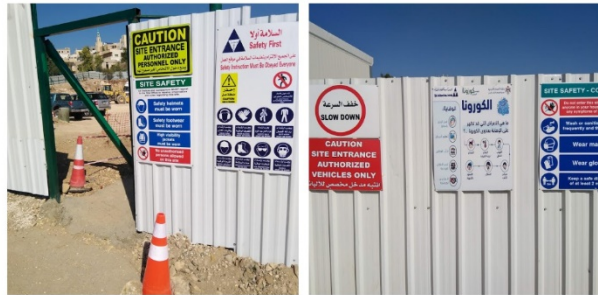
Figure #3: Adequate disinfection stations were secured in the workplace at the entrances and exits; and Publications on prevention and control of the spread of the COVID-19 were distributed in all project facilities. Photo credit: Odai Tawalbeh, 11/18/2020
