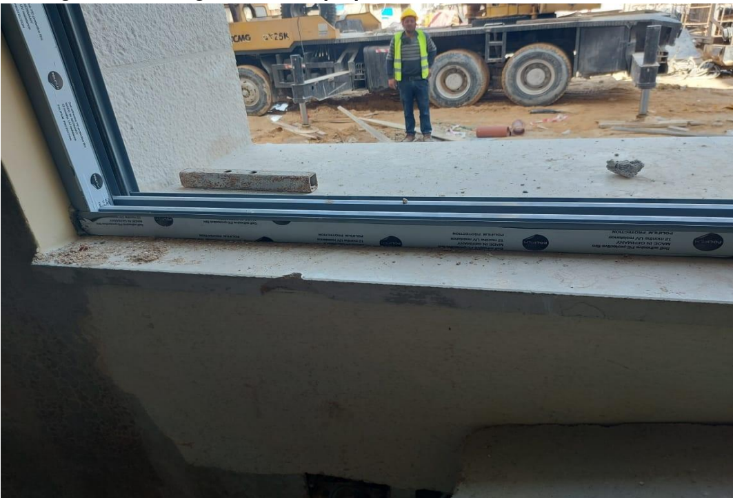
Broken window sill
