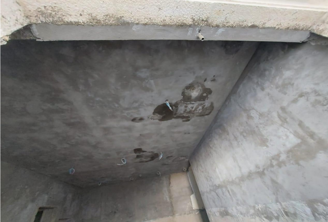
Leakage at the ceiling of the multi-purpose hall
