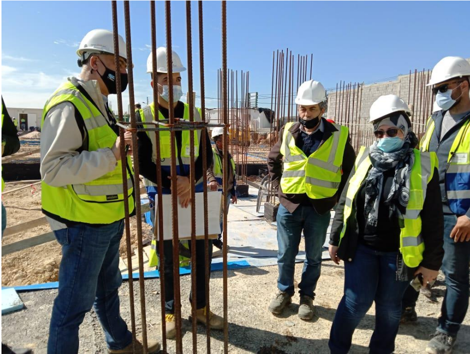
Eng. Hasan Shaqboua Discussing the main issues in the site, including the boundary walls and the actions taken to fix the borders of the school plot.
