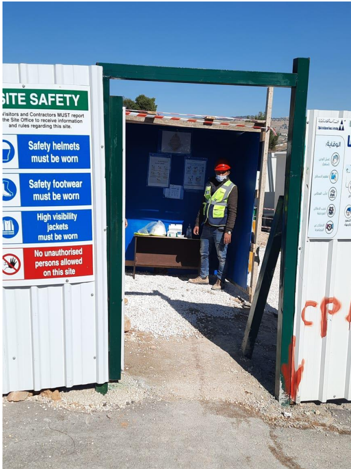
Temperature check and signing visitors' attendance sheet at the entrance of the site, complying with Covid-19 Protocol
