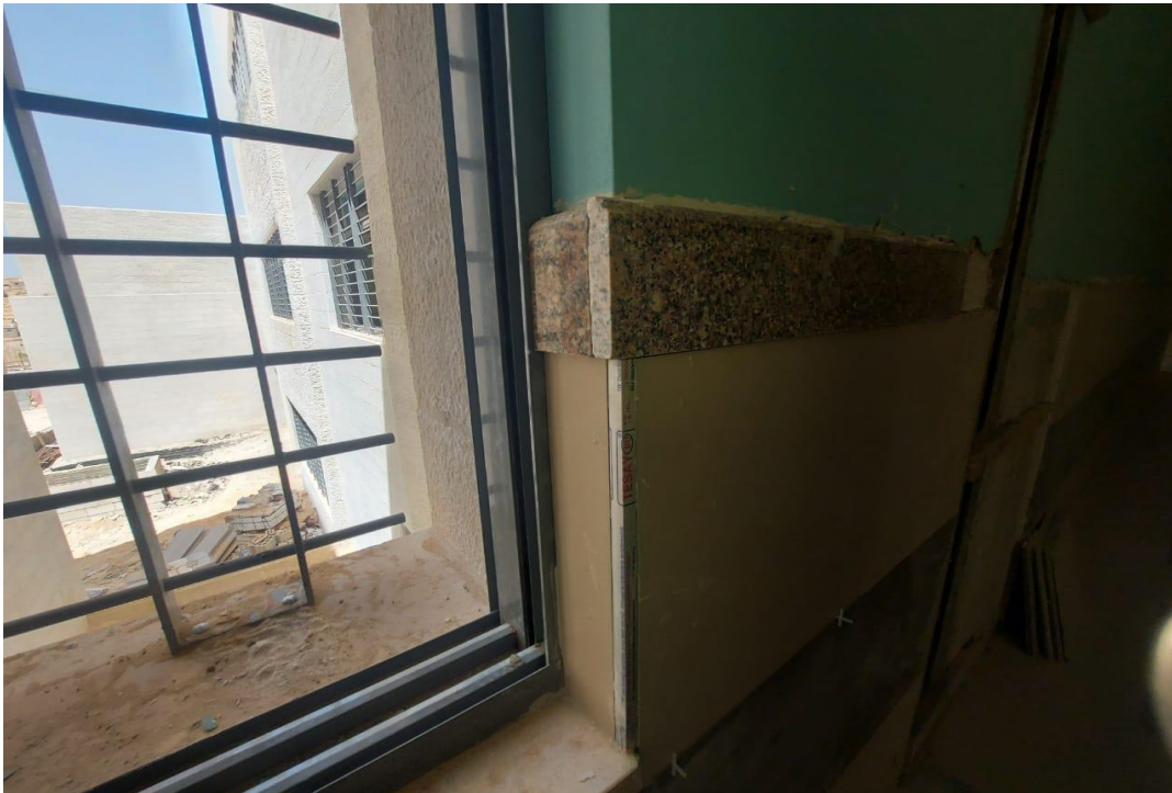
Wrong installation of granite coping
