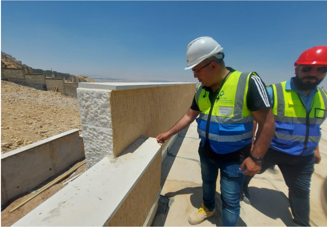
Broken stone coping
