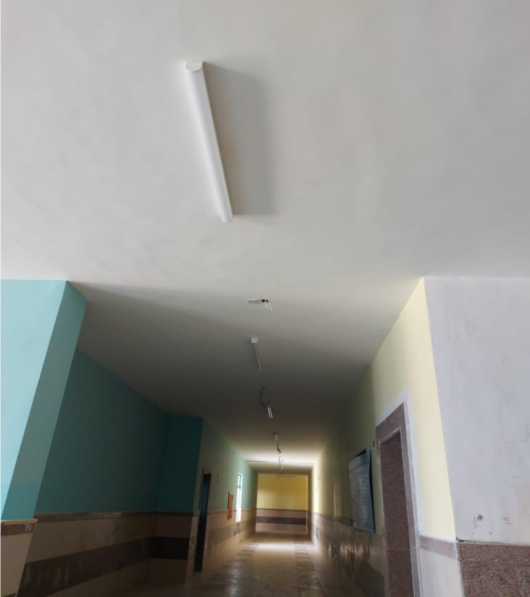
Waving in plastering of ceiling
