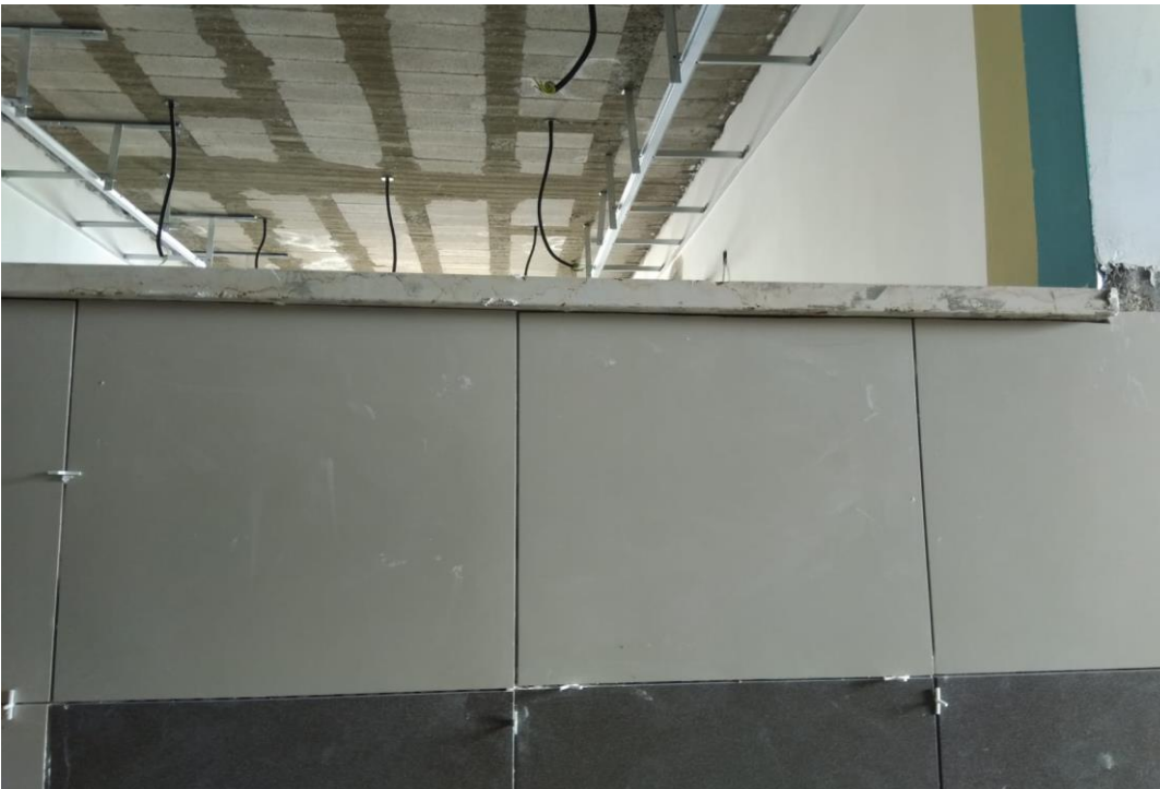
Variations in the levels of window sills
