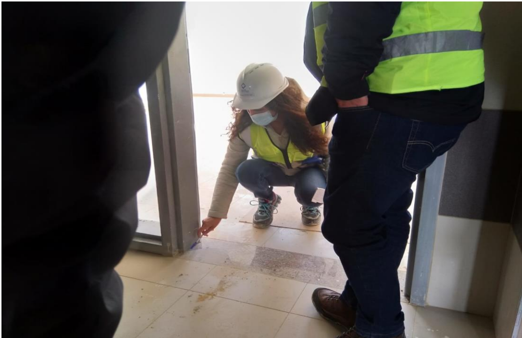
Defects in the threshold
