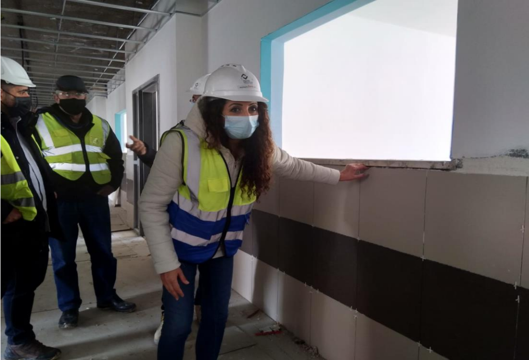
Variations in the levels of window sills
