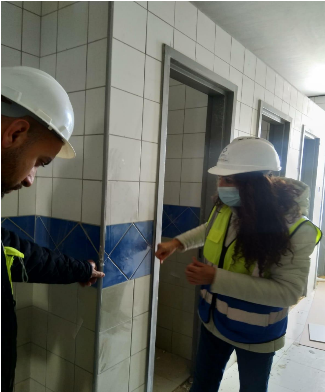
Defects in wall ceramic tiles
