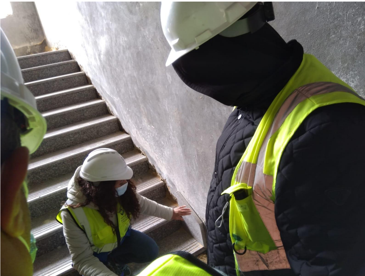
The team inspected the details of the inclined granite skirting for the staircase and insured that the installation is acceptable
