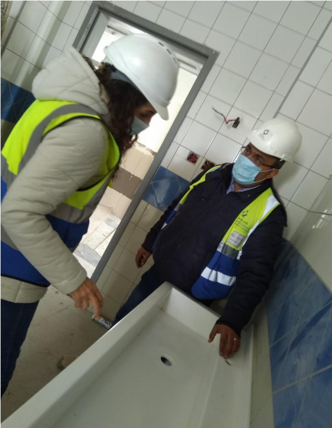
The team inspected the installed wash trough sample and found it acceptable (figure:09 & 10)
