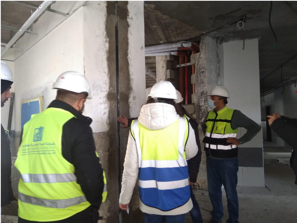
Inspecting the execution of the internal expansion joint and discussing with the Contractor the architectural detail between the false ceiling and the internal expansion joint
