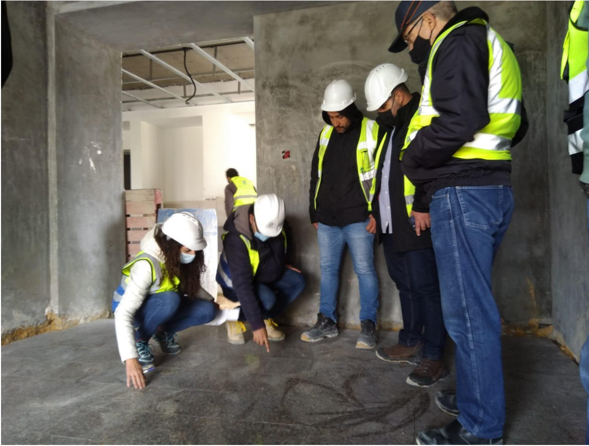
The team inspected the granite tiling at the staircases landing and observed acceptable quality
