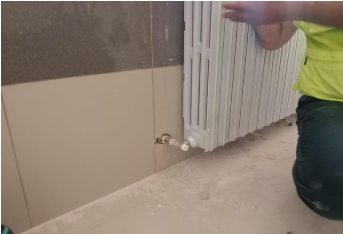
Broken tiles around the radiator connection
