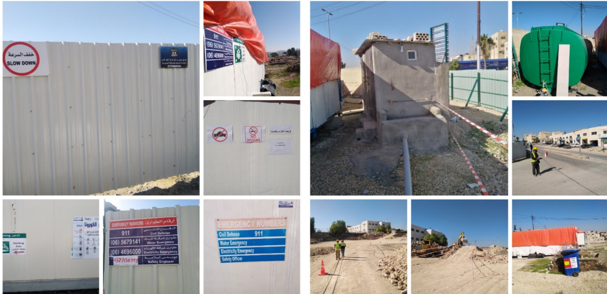
Figure #6: Safety signs and emergency contact numbers available. Publications on prevention and control of the spread of the COVID-19 were distributed in all project facilities. Photo credit: Odai Tawalbeh, 12/1/2020
