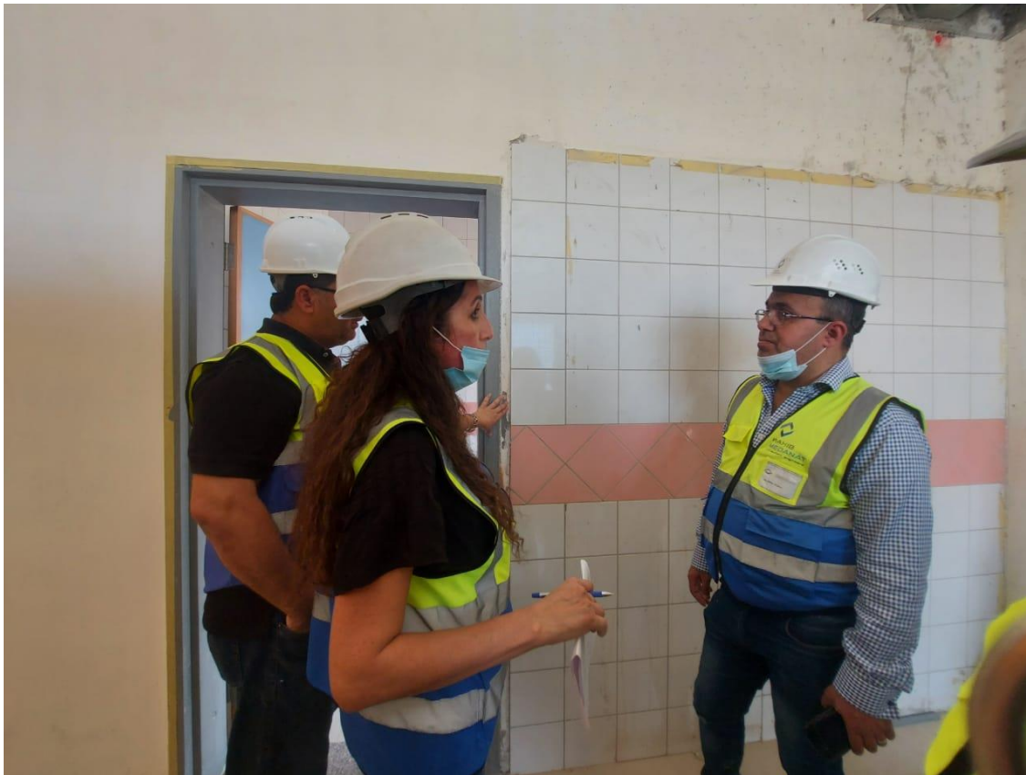
The team inspected the wall tiles and the relation with the door frame at the child care at the (KG) area
