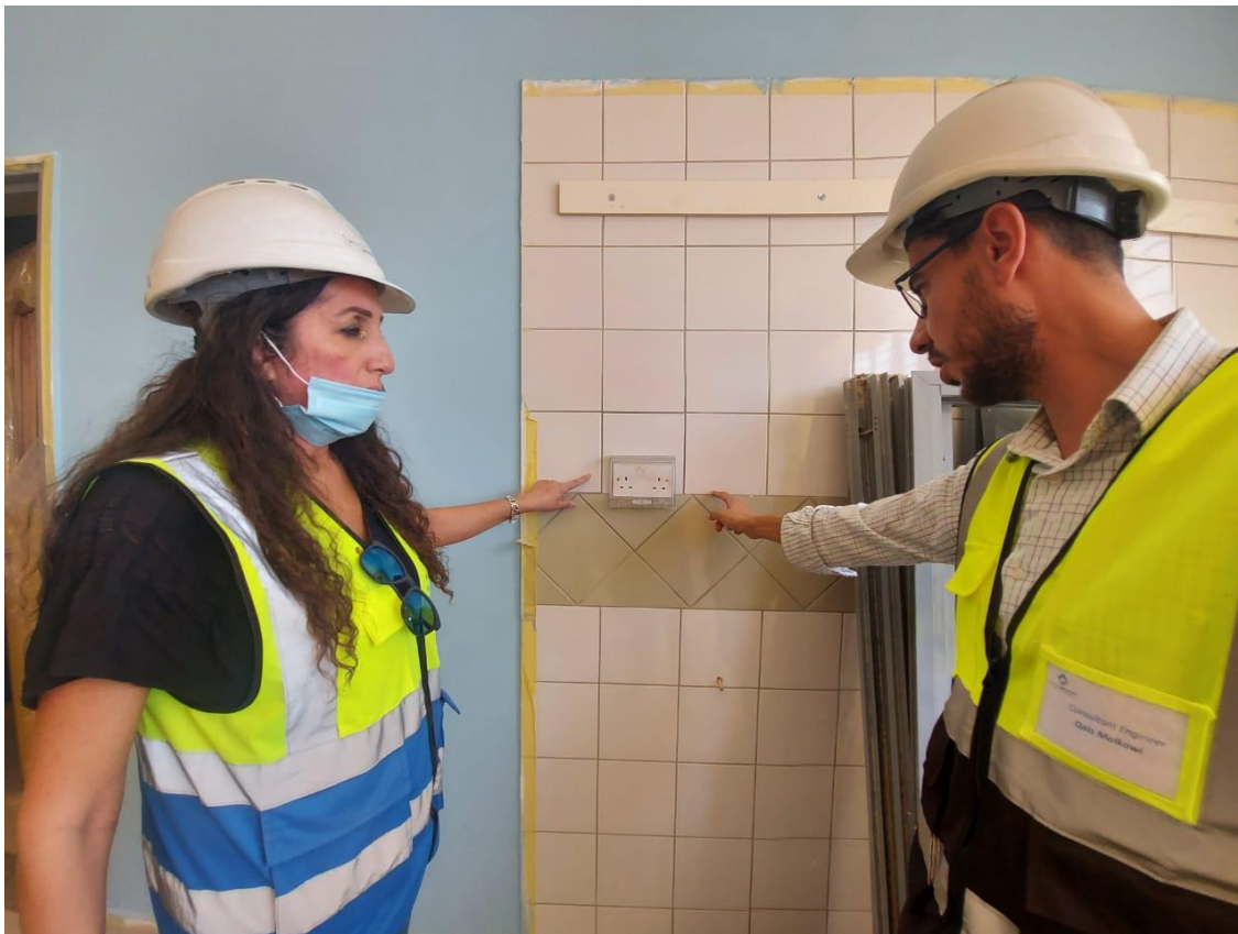
The team inspected the installed sample of electrical socket with cover at the (KG) area and approved it based on the approved workshop drawings
