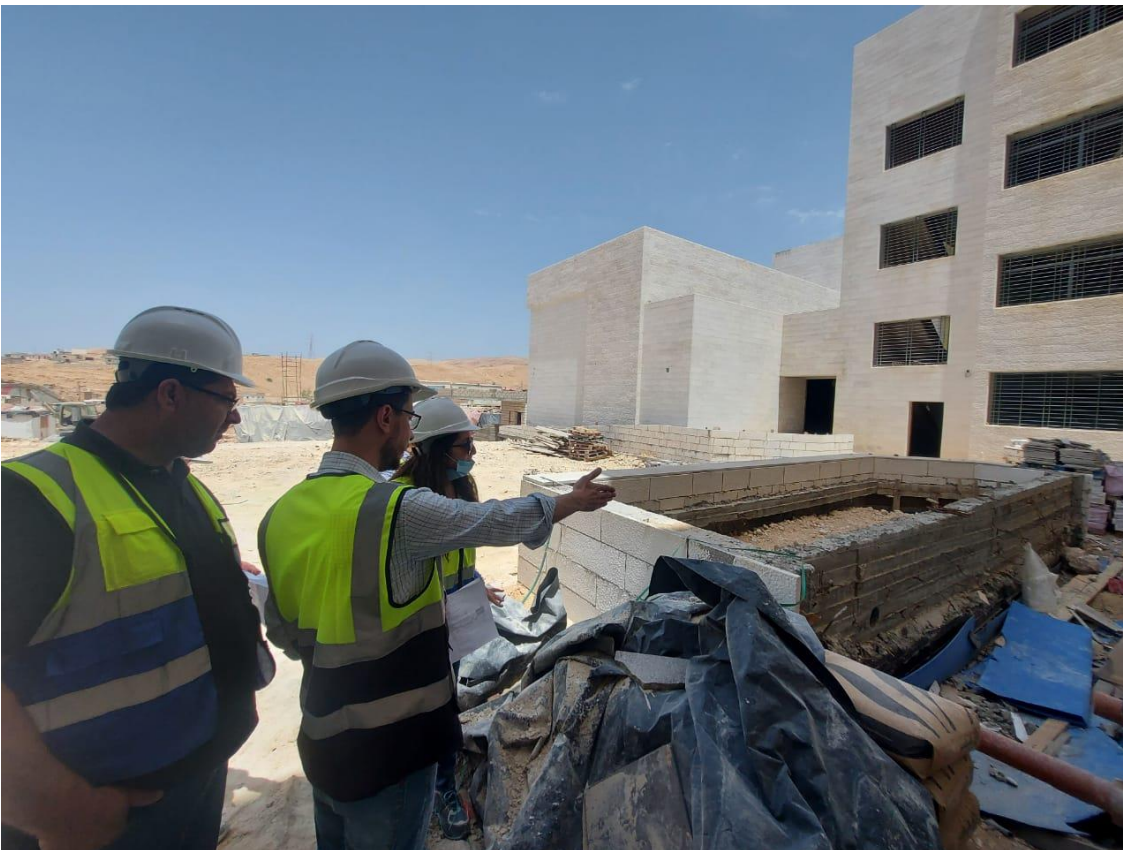
The team discussed with the Contractor the details related to the execution work of the external ramp adjoining the main entrance and observed variation from the approved workshop drawings
