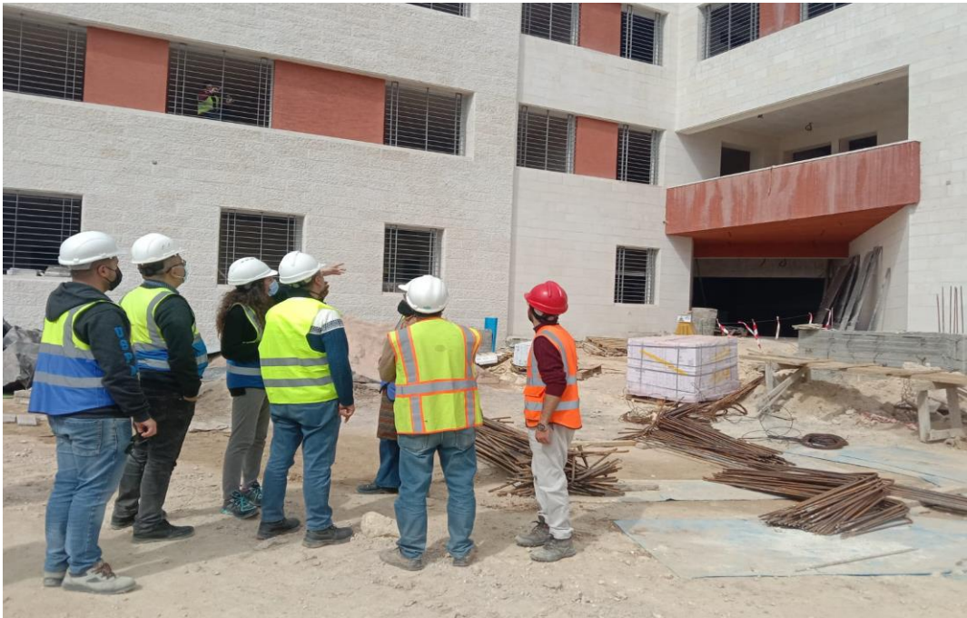
White color appears on the surface of external plastering
