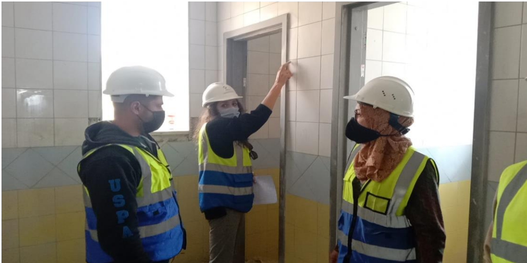
Defects in the wall ceramic tiles cutting adjoining the door frames
