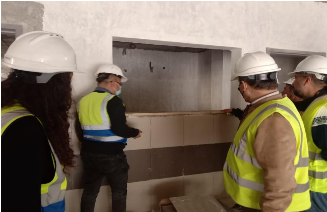
Wrong level of the window sills
