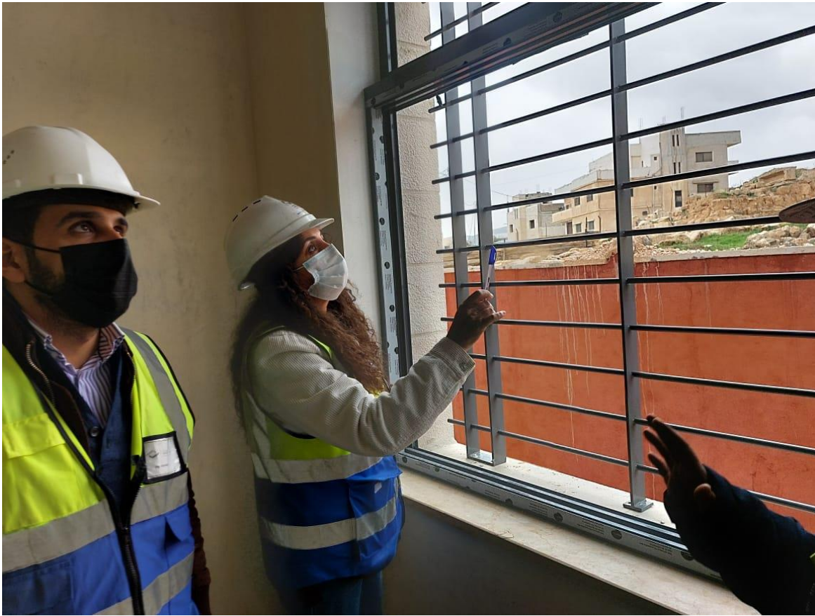
The team inspected the fixation of the steel protection screen and observed corrosion in some parts
