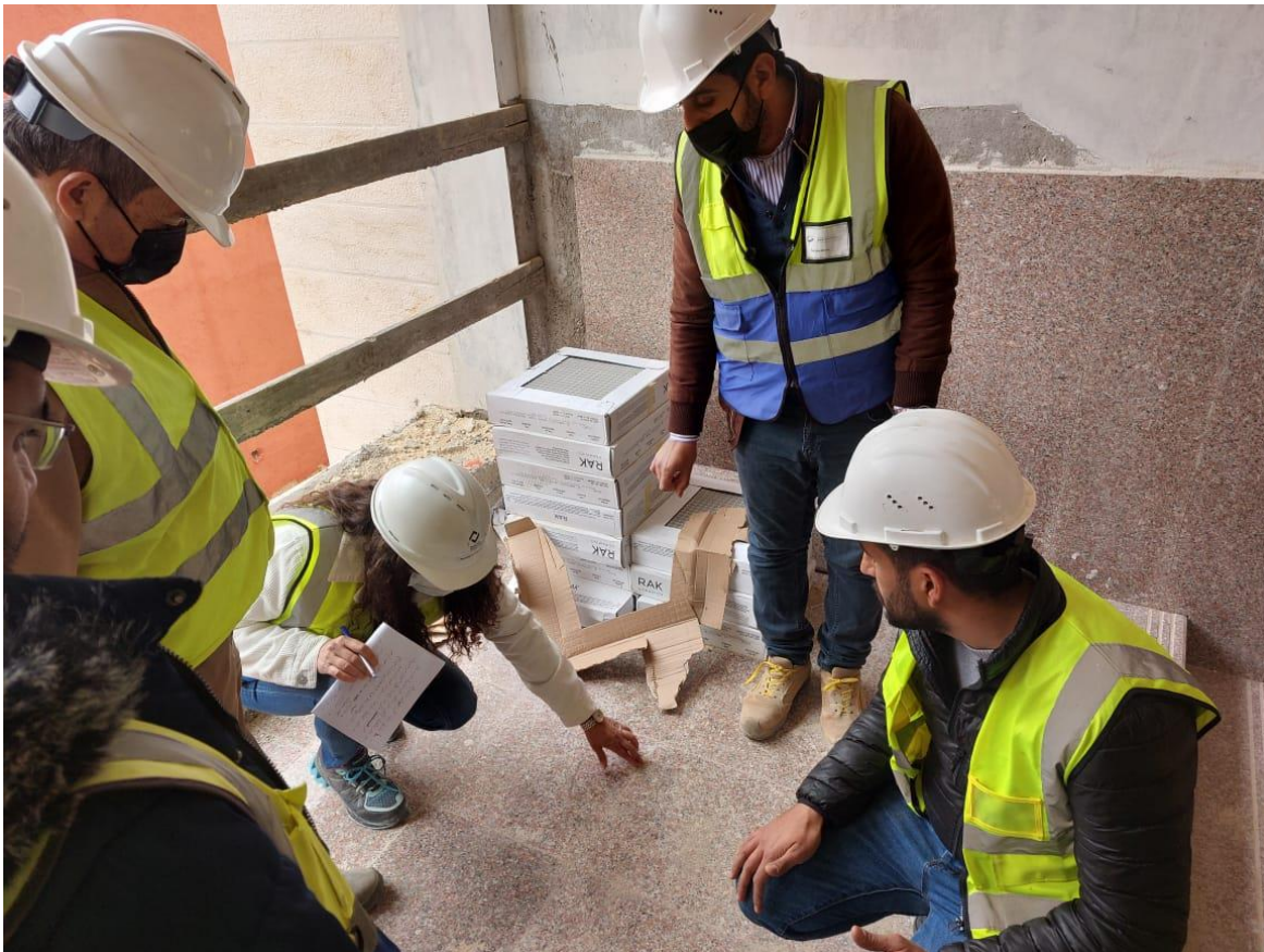
The team observed that the granite tiling for stair landing is not rectified by the Contractor and the teething is still visible
