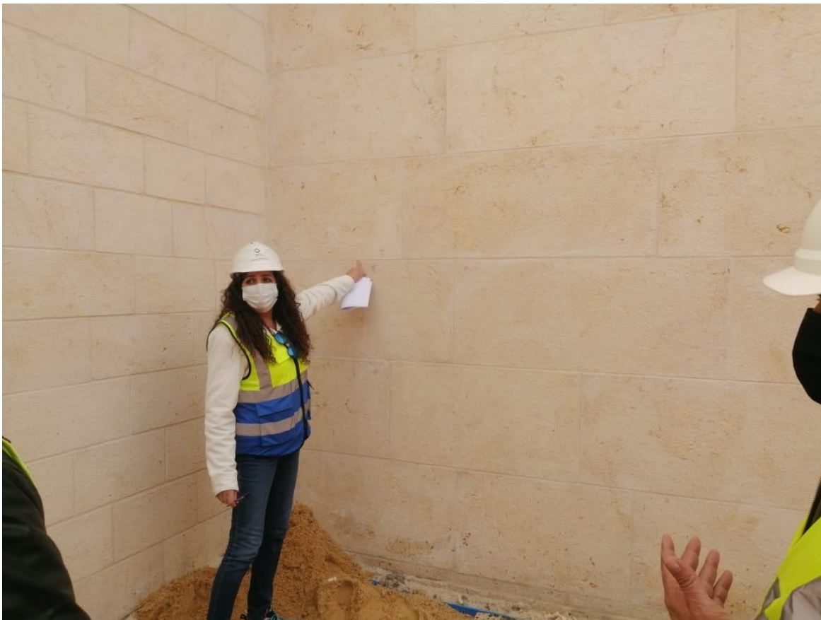
The team observed that the Contractor tried to rectify a number of stones by covering the defects with cement mixes, but that is not accepted
