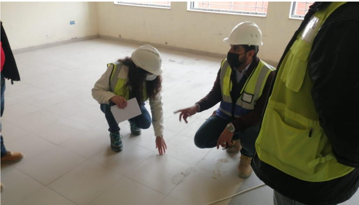
The team observed minor teething in some parts in the porcelain floor tiles and requested the Contractor to rectify
