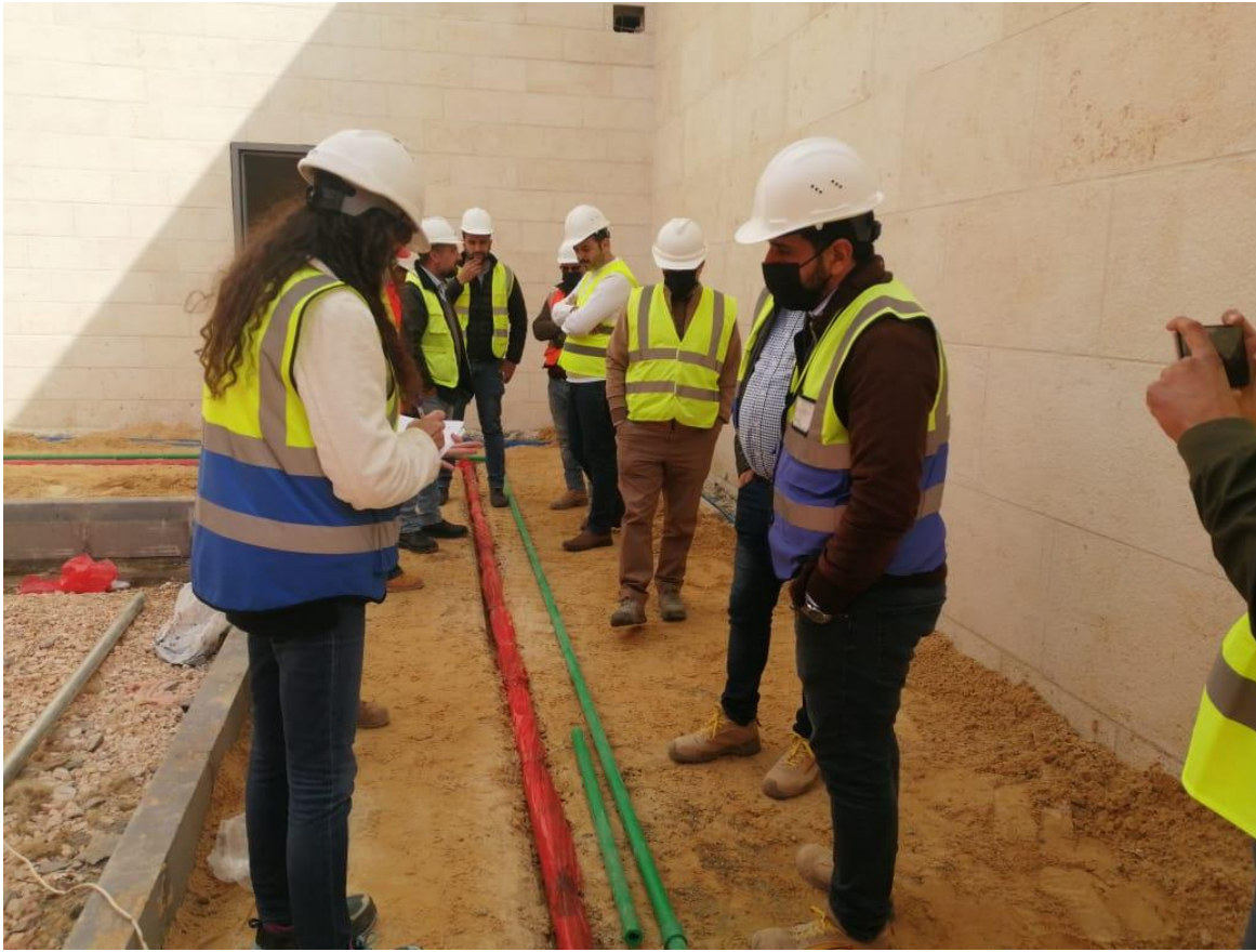
The team observed the execution of water pipes under the external sidewalks
