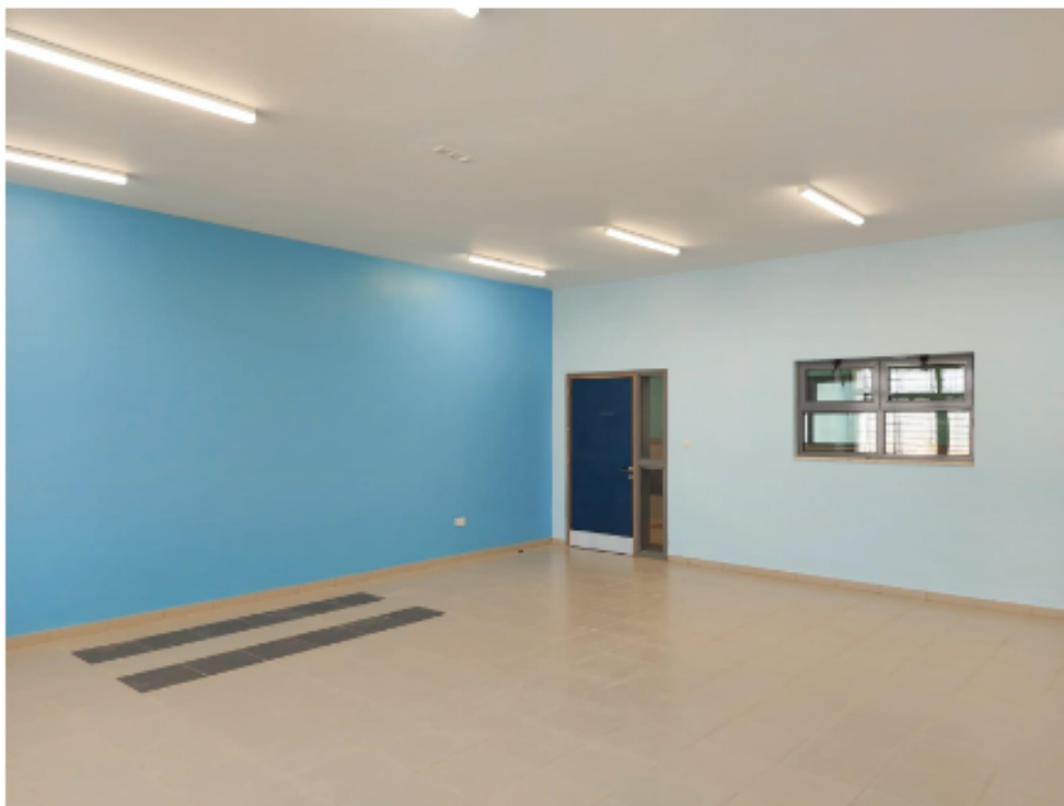
The team observed that the Contractor finishing painting works at the classrooms and corridors
