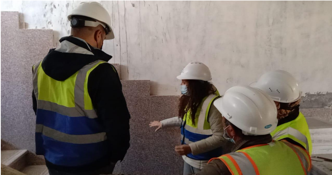
Defected granite for the staircases
