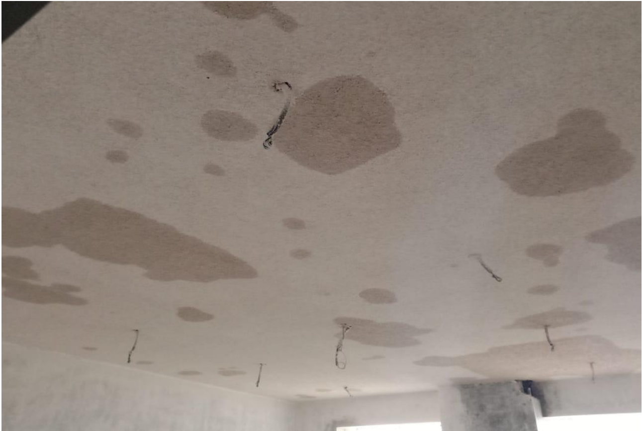
Water penetration from the pumps room at the roof
