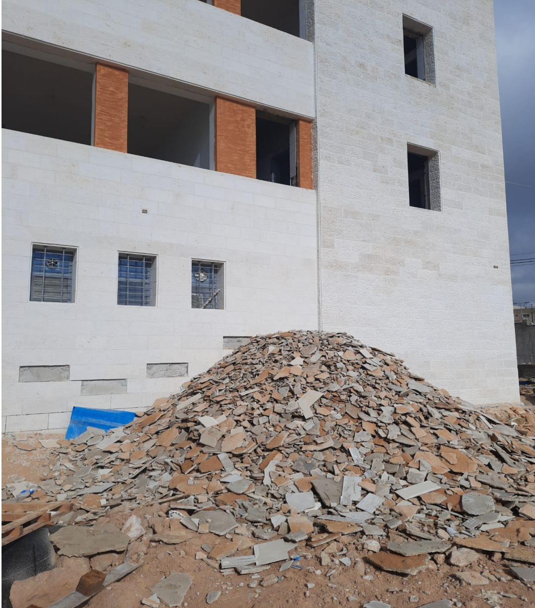
Defected stones and cumulative debris
