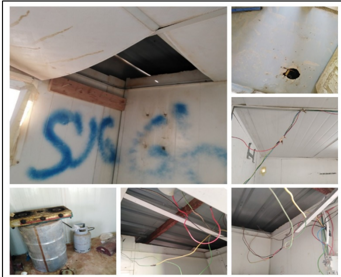
Figure #5: Unsafe (damaged) workers trailers that were observed on site; Hanging and exposed electrical wiring; Dirty Gas Stove stained while cooking; and Gas stove cylinder that was observed in a poorly ventilated room. Photo credit: Odai Tawalbeh, 1/25/2021
