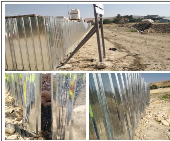
Figure #4: No safety signs along fences on site as well as a part of fences were damaged due to the accumulation of excavation materials near them on site. Photo credit: Odai Tawalbeh, 1/25/2021
