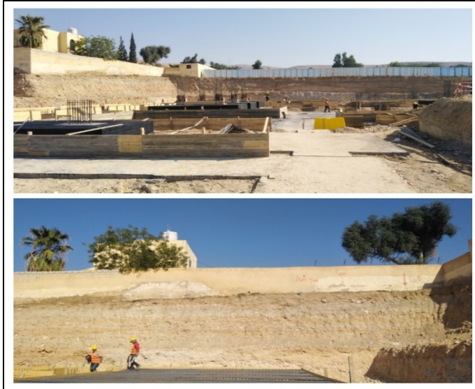
Figure #6: Dangerous Condition: A weak boundary wall of the neighboring residential building that already has no footings was observed on site; risk of collapse which could lead to the serious incident. Immediate Action Required. Photo credit: Odai Tawalbeh, 1/25/2021
