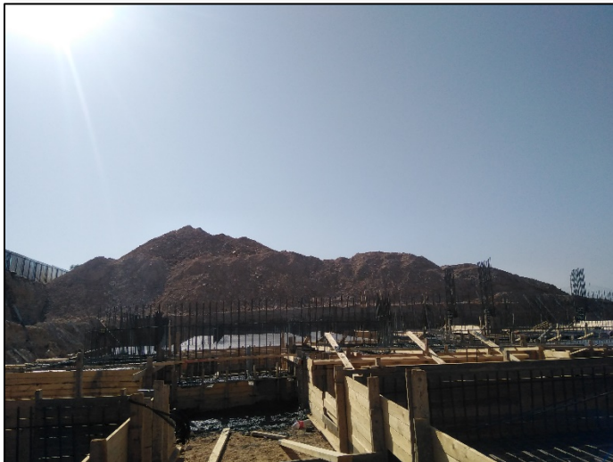
Figure #7: Excavation materials that were accumulated near fences on site. Photo credit: Odai Tawalbeh, 1/25/2021
