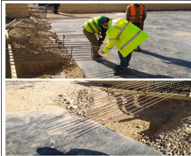
Figure #3: A protruding steel reinforcement bars that were observed on site along with the corrective action taken immediately from the contractor side by providing all steel bars with safety mushroom caps. Photo credit: Odai Tawalbeh, 1/25/2021
