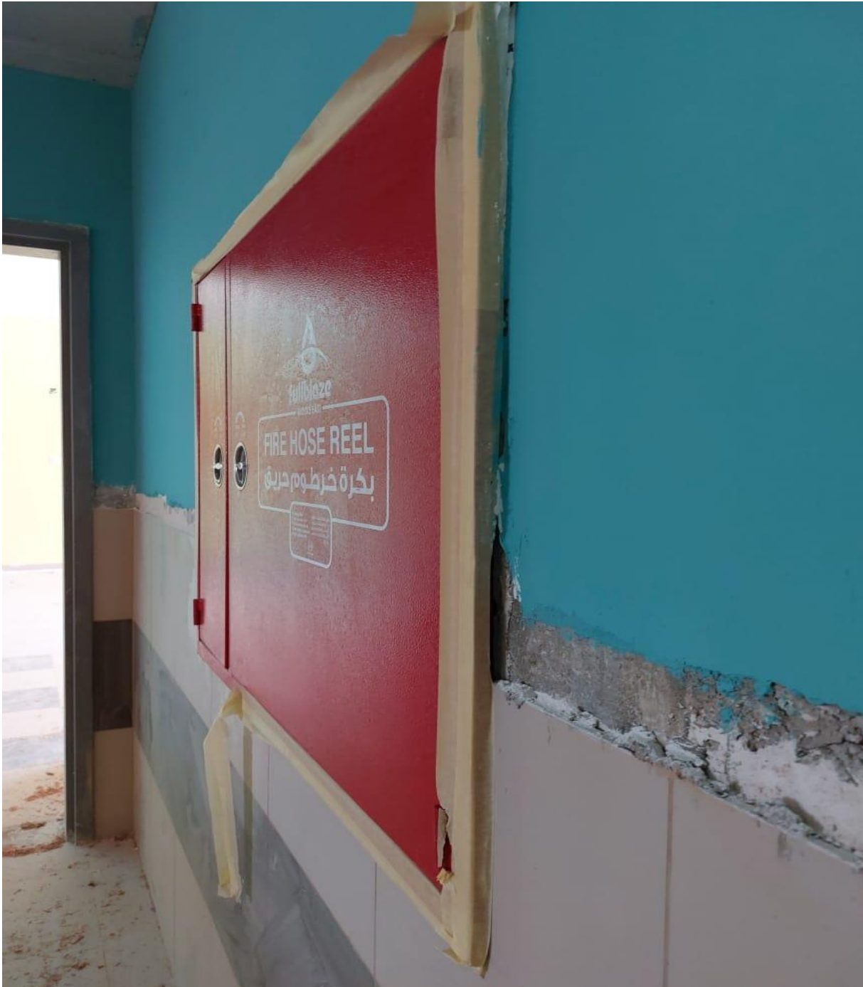
Gaps between the cabinet frame and the wall
