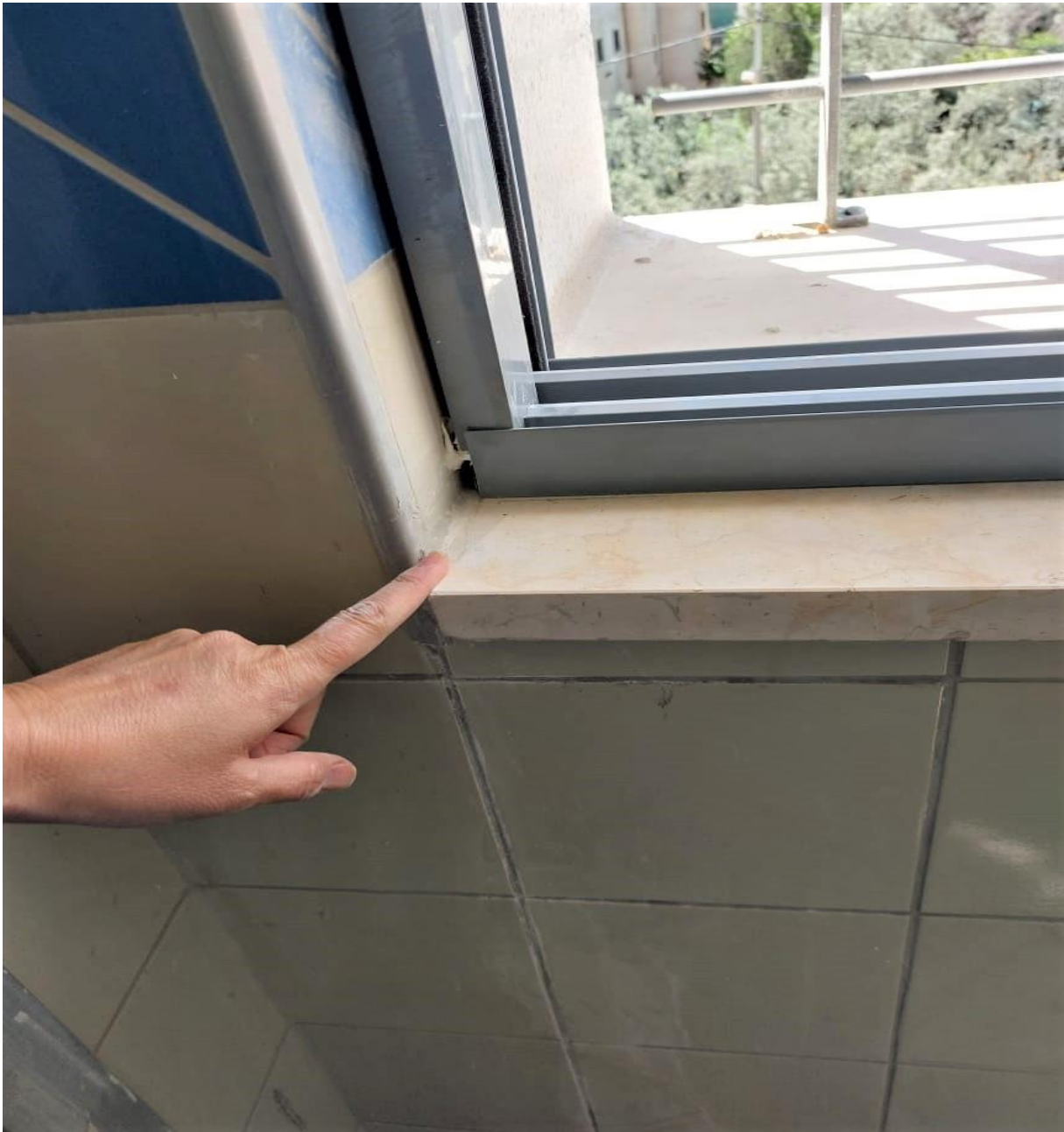
Wrong dimension of aluminum sections
