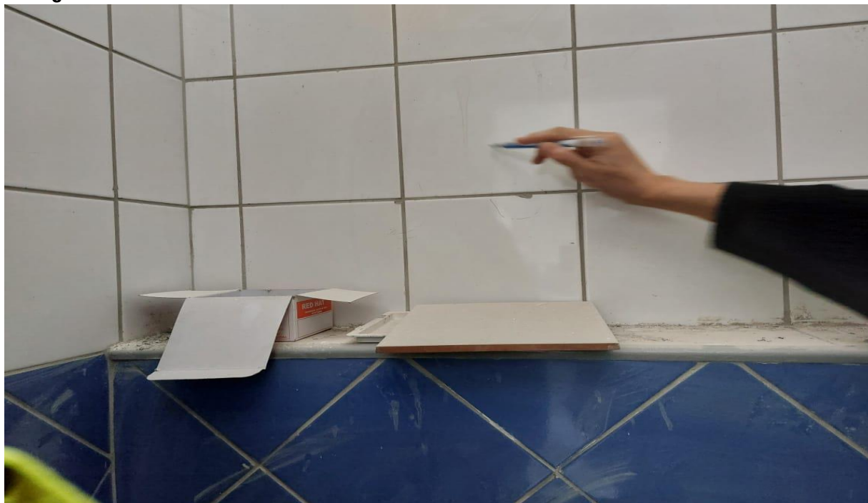
Broken ceramic tiles
