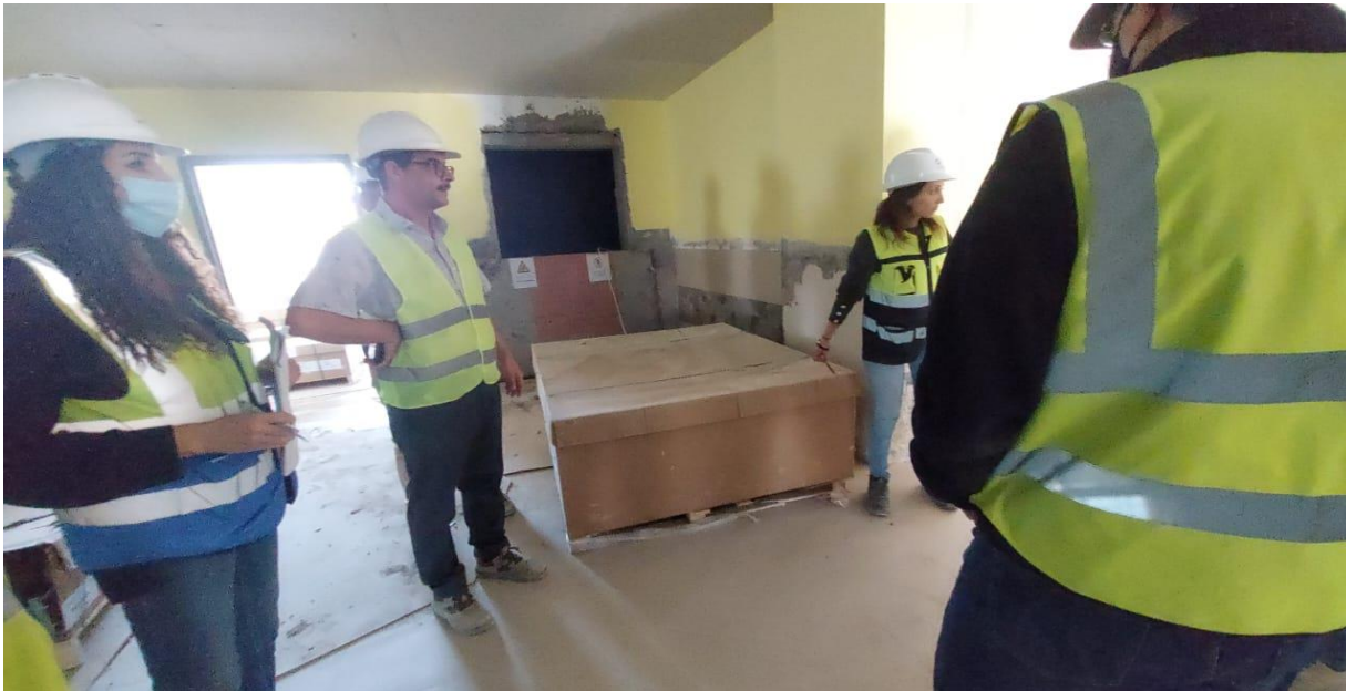
Inappropriate storage for the elevator equipment
