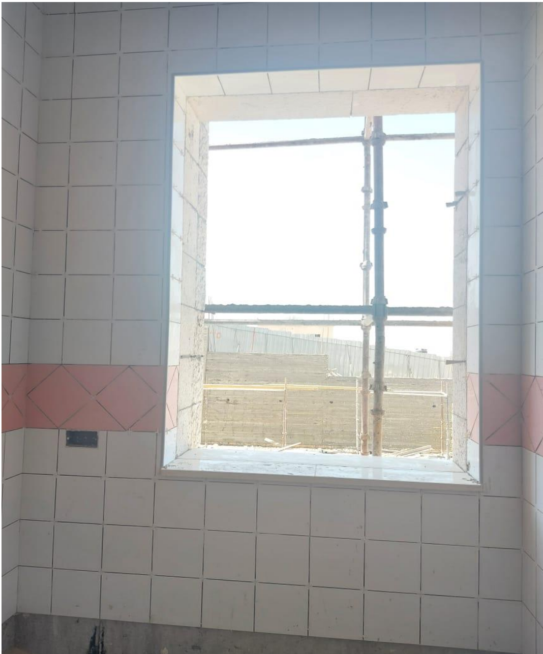
Defects in installing wall tiles
